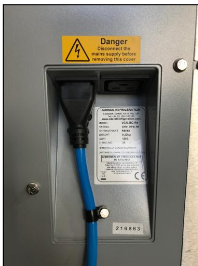
Figure 3: Mains connection point
